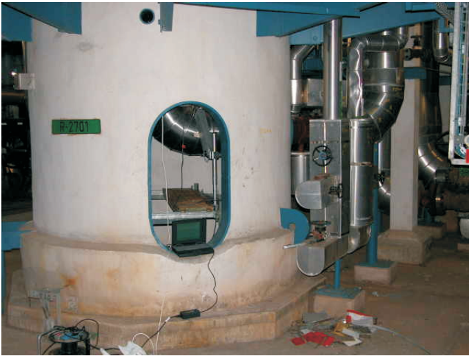
Skirt of the reactor with 10" feed pipe
